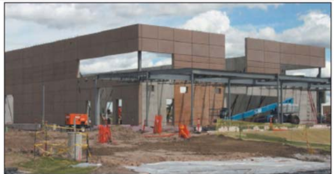
A 32,000 square-foot public works facility — under construction at Hess Road and Tammy Lane — will be ready for move-in in May 2015. Photo by Chris Michlewicz
